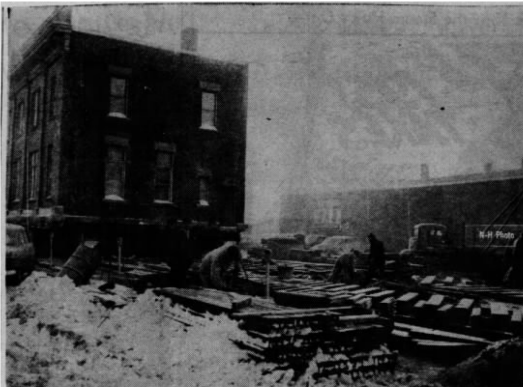
PREPARING THE TRACK —Workmen for the Frank P. Noe Company, Chicago, are shown as they prepared the track for moving the Connor Lumber and Land Company office building, 400 S. Central avenue, to its new location half a block west on Fourth street. The first phase of the moving operation—pulling the brick building back to the point where it will be turned at right angles to its old position—was completed late yesterday afternoon before a large and appreciative audience of sidewalk superintendents. The actual moving job is expected to be completed Saturday.
