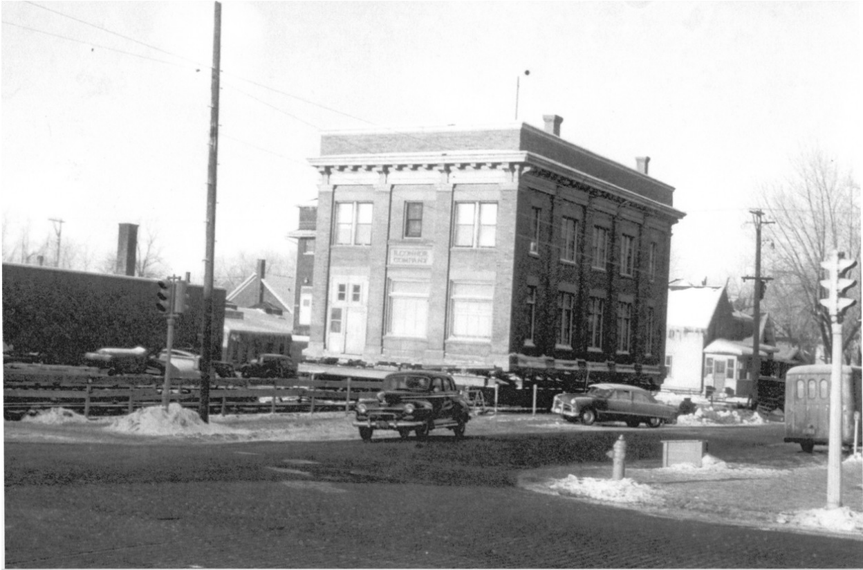
The R Connor office building being moved from 400 South Central Avenue to 108 W 4th Street. Once at its new location the building was rotated so the front entrance now faced north. In this photo, the building has not yet been rotated.
